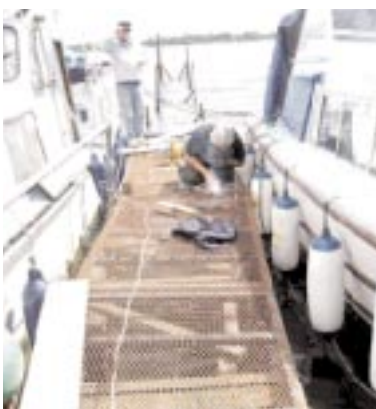
During the 1960s, a jetty was built by the McGarry brothers, who had leased the island from Lord O'Neill, to facilitate visits by the passenger vessel the Maid of Antrim. The McGarry jetty, which is located at the south-eastern end of the island has now fallen into disrepair, but to facilitate repair operations to the summer house, members carried out temporary repairs to the jetty
